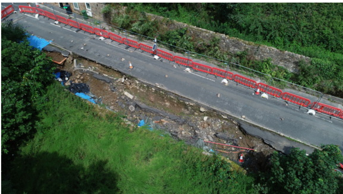
Drone photograph of the landslip at Leashaw.prior to removal of debris.
