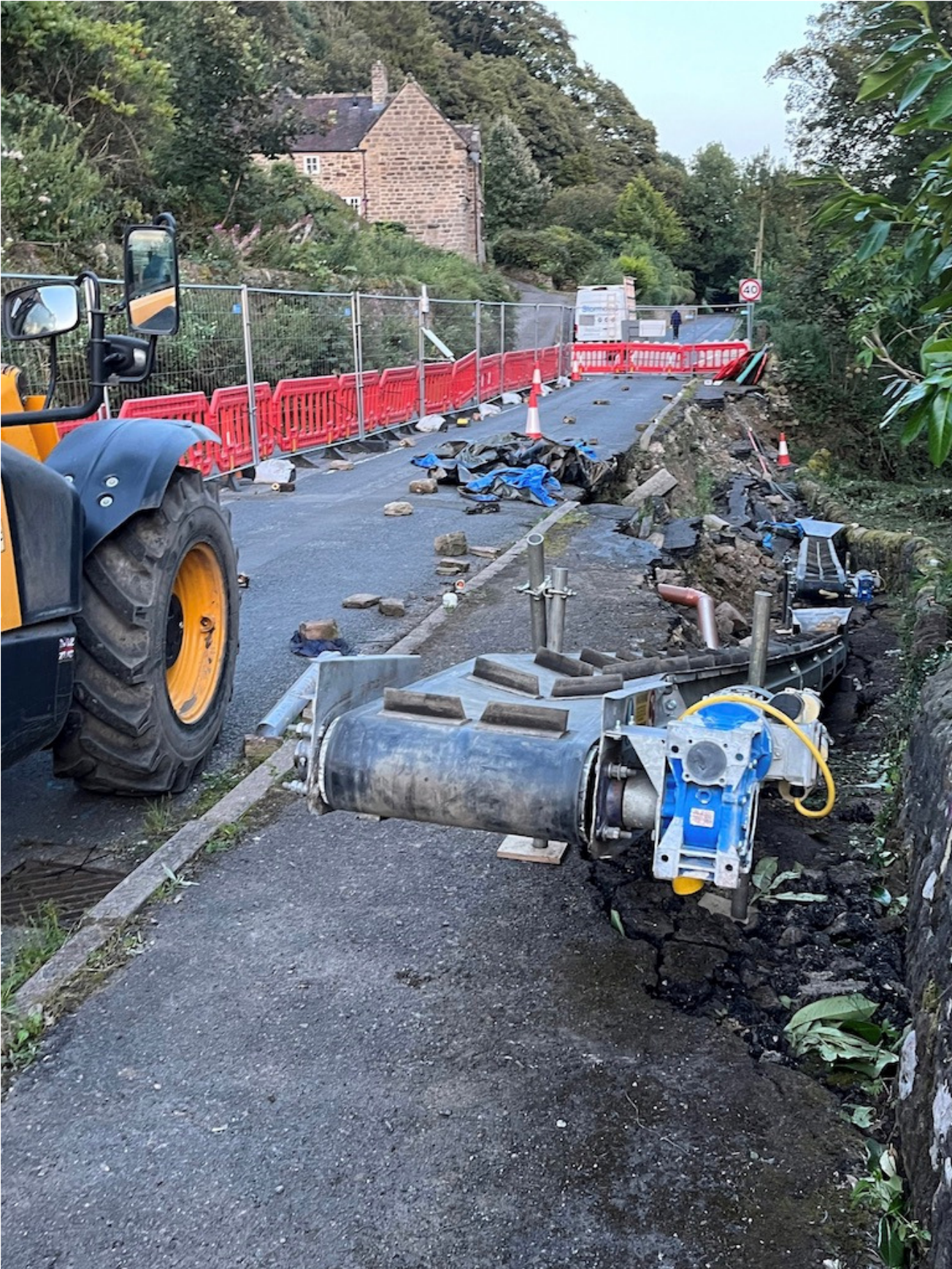
Current state of Leashaw road closure: removal of collapsed wall from the landslip.
